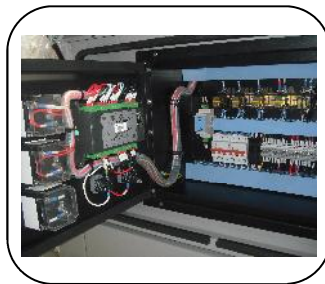
Wiring and protection in accordance with AS3000 and AS3010. Robust, clear labelling system with comprehensive schematic drawings.
